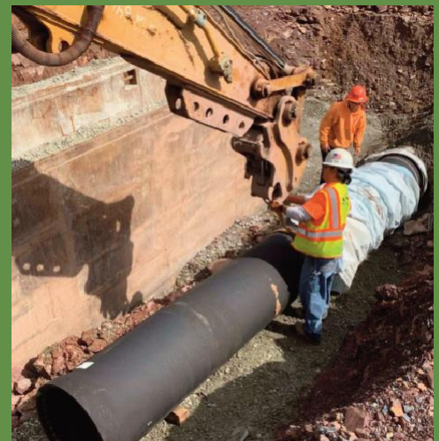
Brodhead Creek Regional Authority - Tannersville Tank and Pump Station
